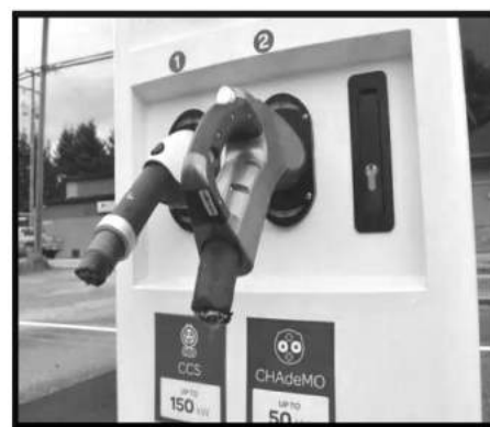
Cables easily severed at electric vehicle charging station
